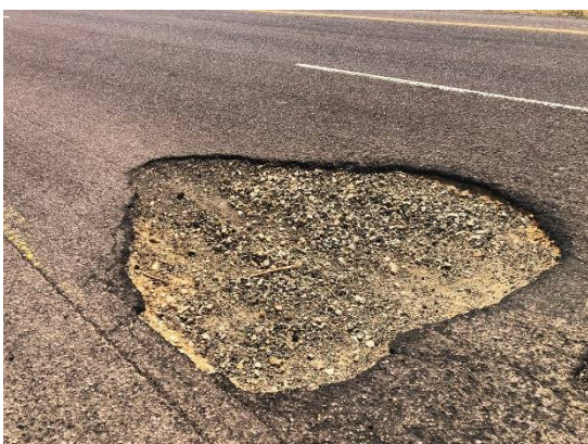
Left: The evil pothole. It is deeper than it appears. (all photos ZS4TX)
